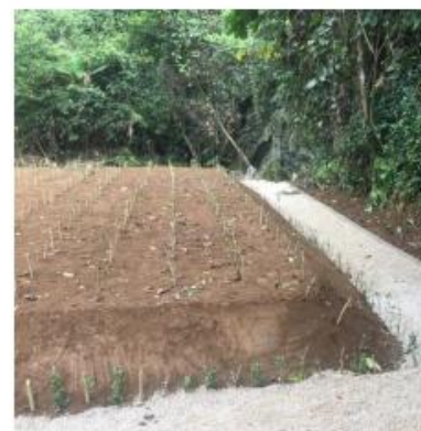
Indigoberry was planted on surface and crushed-stone aggregate road was constructed around
