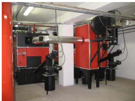
One of the boilers installed in Slanická Osada
