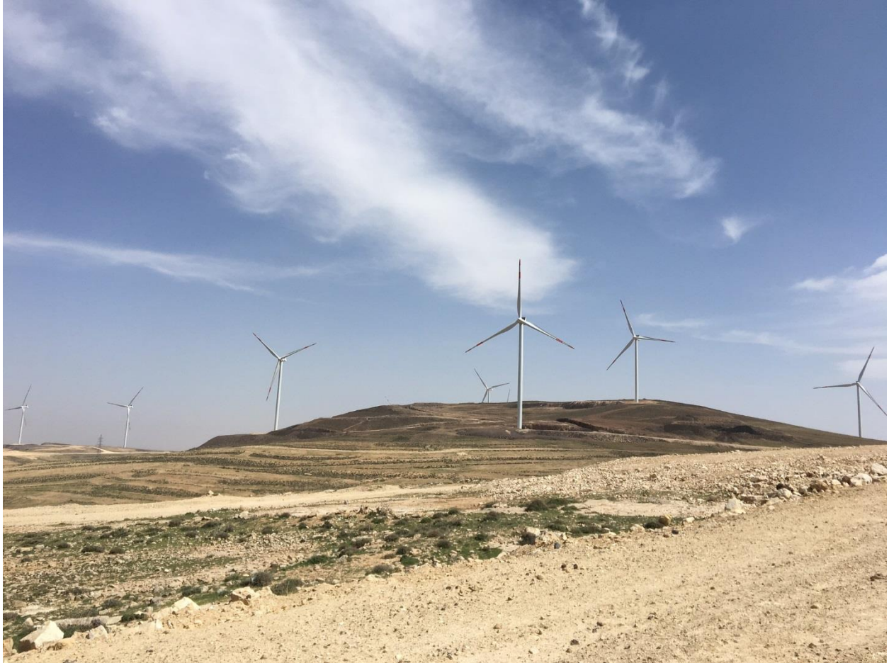
Figure 12.3. Northern part of the Tafila Wind Farm (Source: World Bank staff; Site Visit 03/08/2016)
