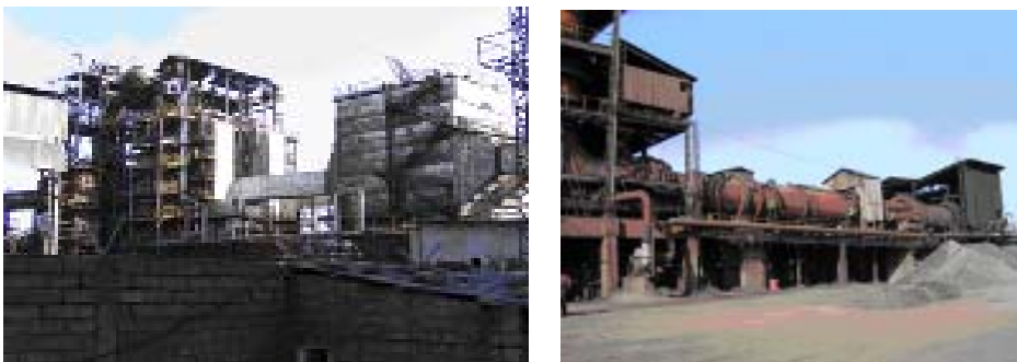
Figures 1 & 2: Waste Heat Recovery Boiler and Kiln
