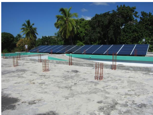
Image 17: Solar panels. Port-à-Piment.
