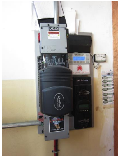
Image 13: Inverter, charger, electronics. Coteaux.
