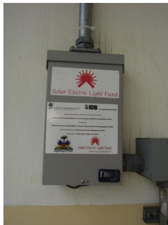
Image 14: DC junction box. Coteaux.
