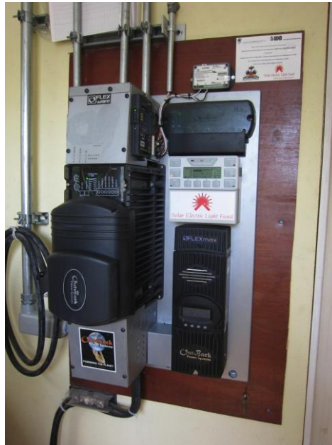
Image 25: Inverter, charger, and electronics. Roche-à-Bateau.
