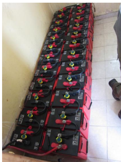
Image 15: Battery bank. Coteaux.
