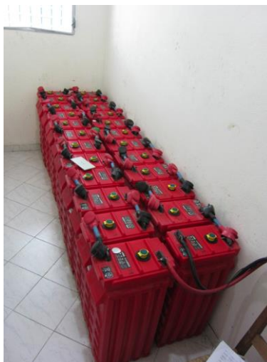
Image 21: Battery Bank. Port-à-Piment.
