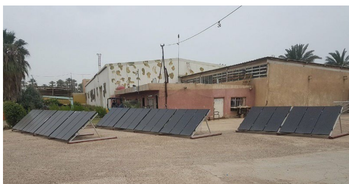
Solar energy unit at Al Mansour Factory – Baghdad provided by the project May 2016
