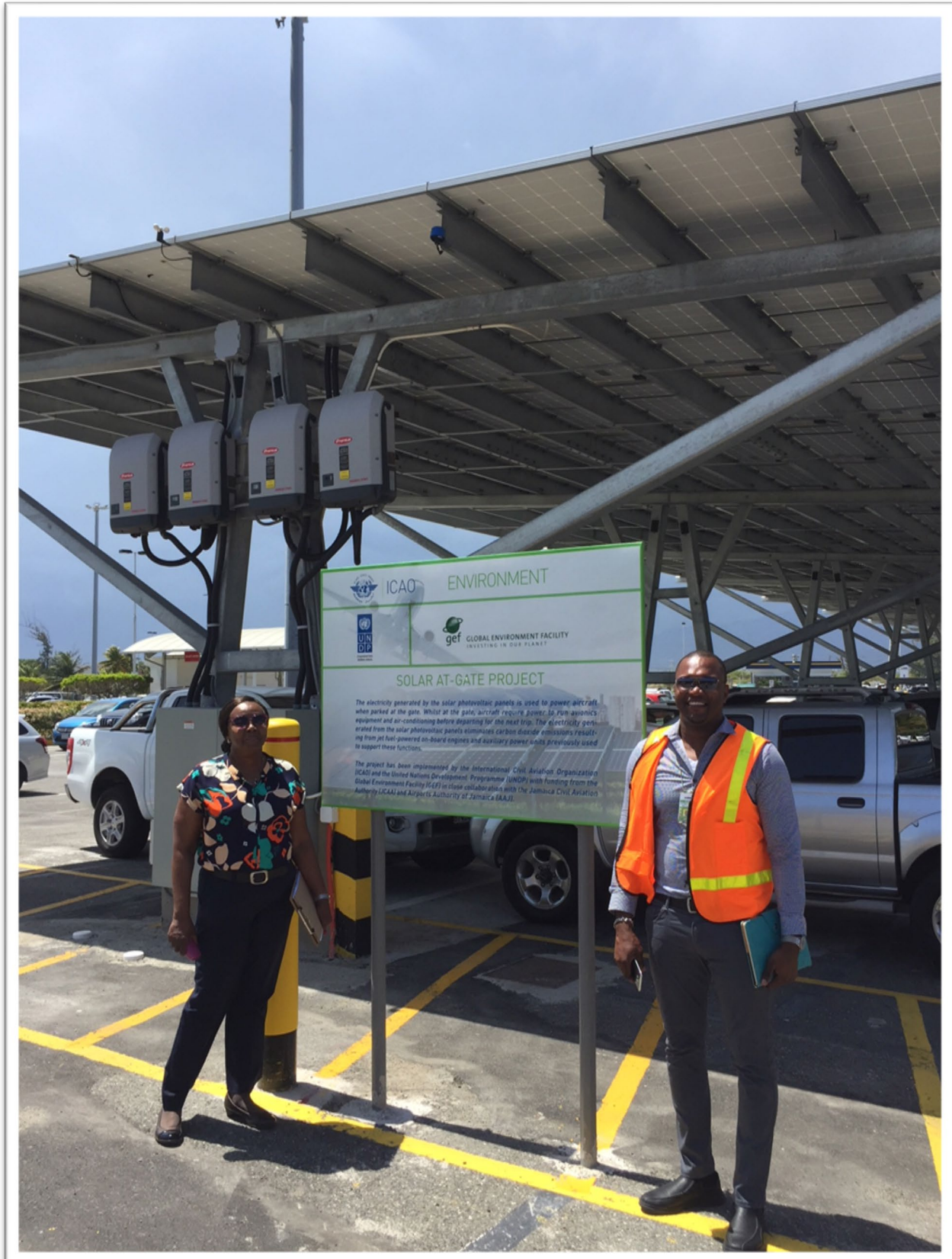
Figure 14: Ms. Althea Roper and Mr. Junior Levene next to 100KW Solar PV array the public parking lot. Note the sign clearly alerting the public of the solar-at-gate project.
