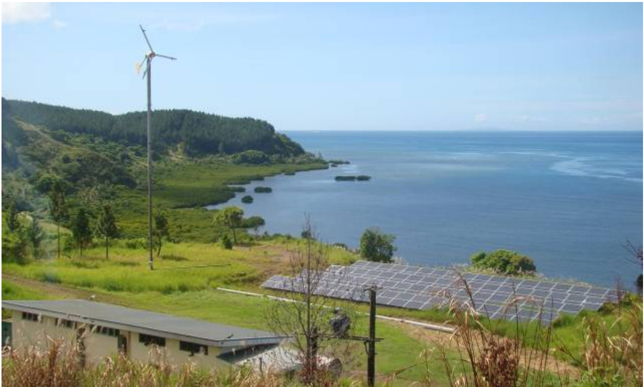
Solar-Wind-Diesel Hybrid System in Nabouwalu, the initial proposed demonstration site for the RESCO project Photograph taken during the final evaluation site-visit in February 2010
